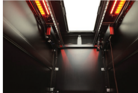
Internal view of IT space - front door
