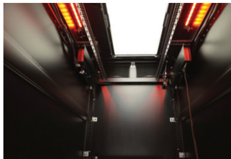
Internal view of IT space - front door
